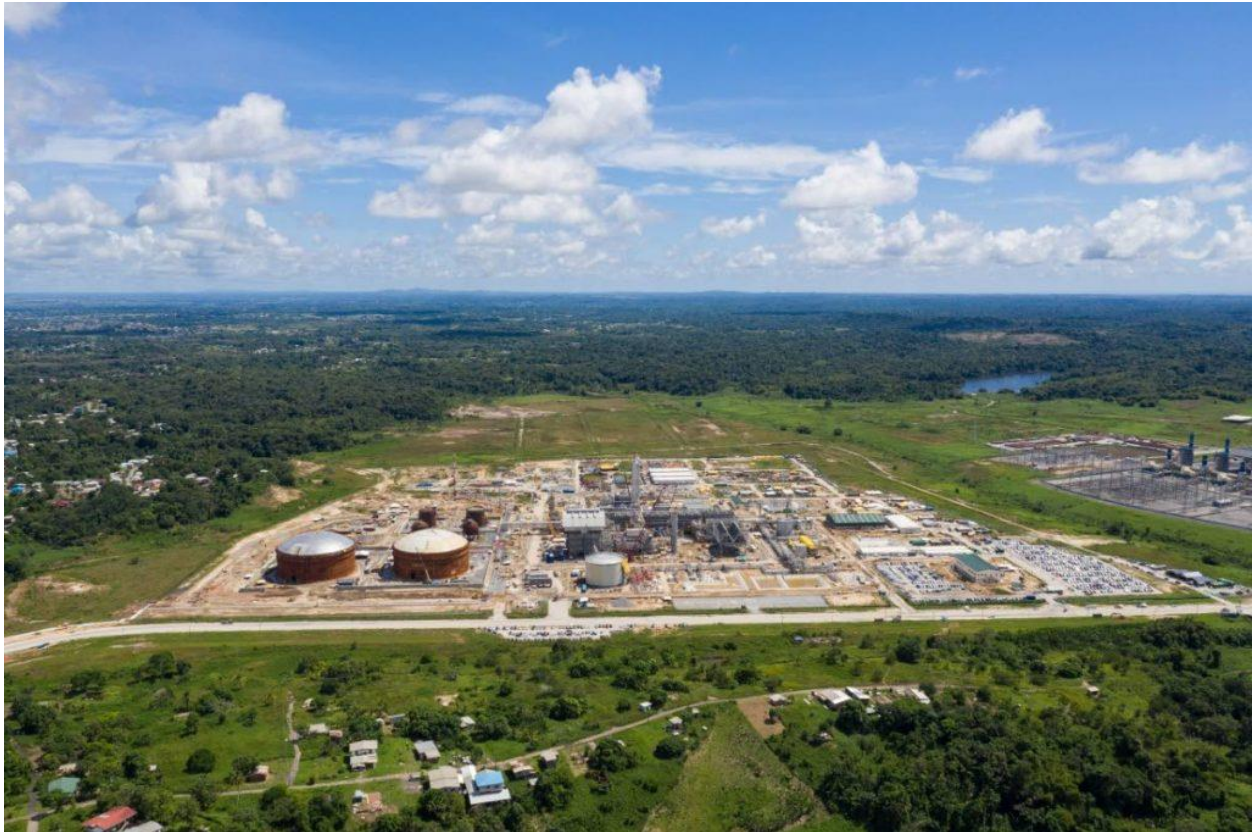
The CGCL plant under construction at Union Industrial Estate. Photo courtesy National Energy Corporation. –
