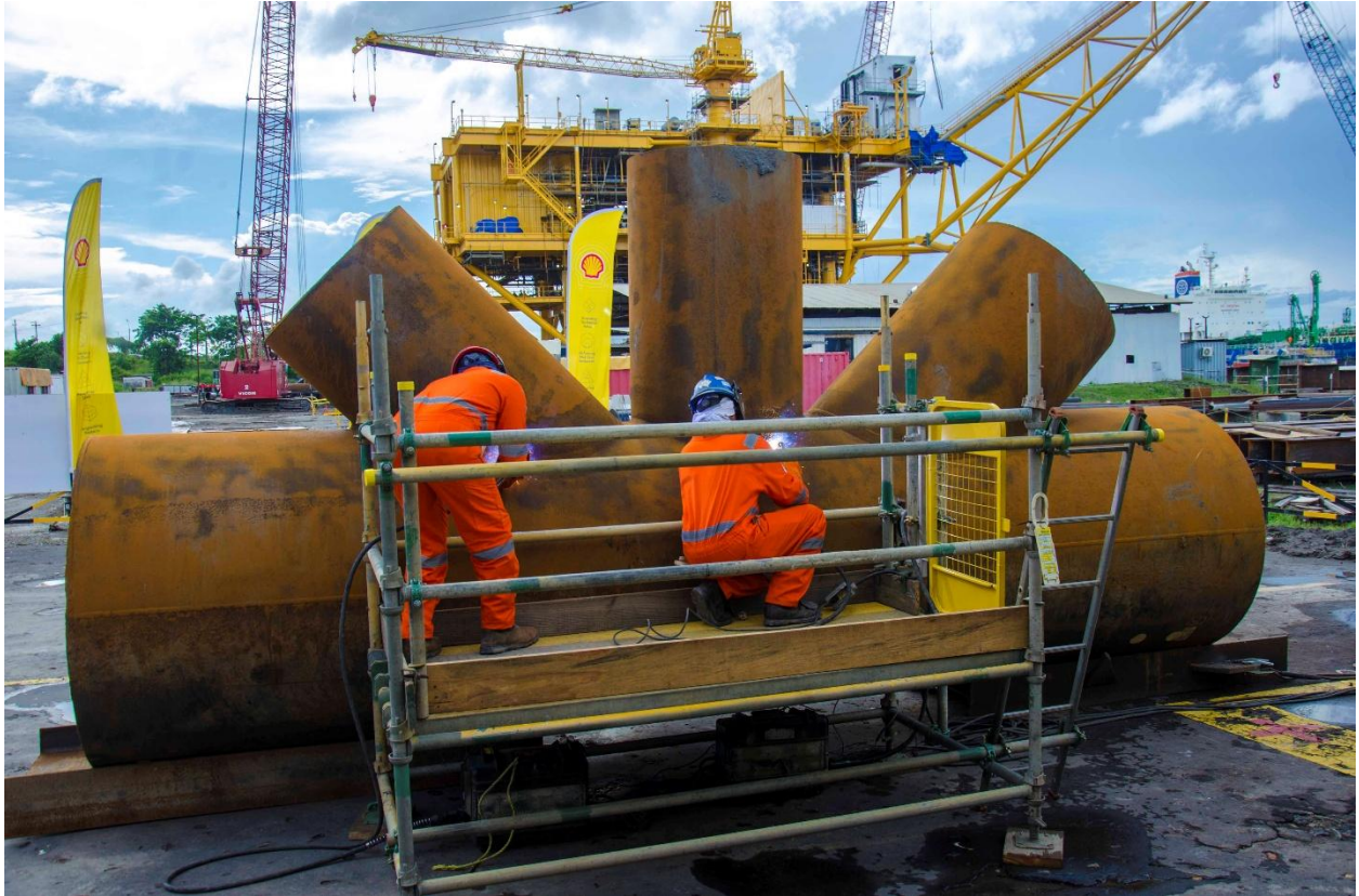
The ceremonial simulation of steel cutting to signal the commencement of the local fabrication phase for the Manatee Project, at the TOFCO Yard, La Brea Industrial Estate.
